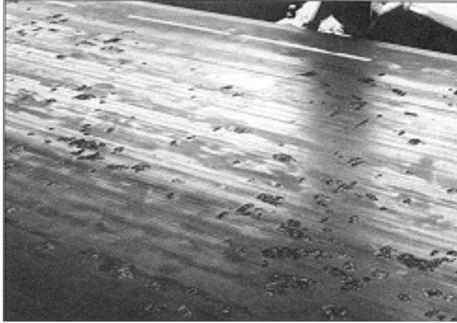
Figure 12 Belt damage due to impact.
